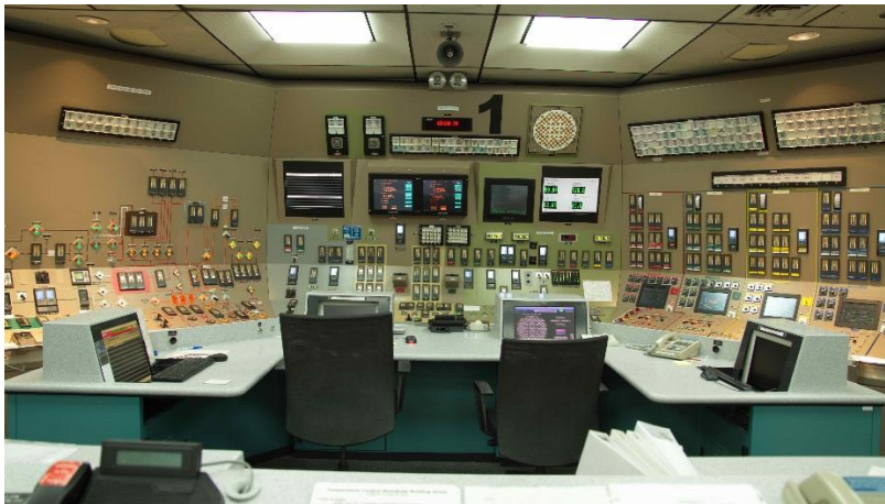
Figure 2: Existing PVNGS Control Room
