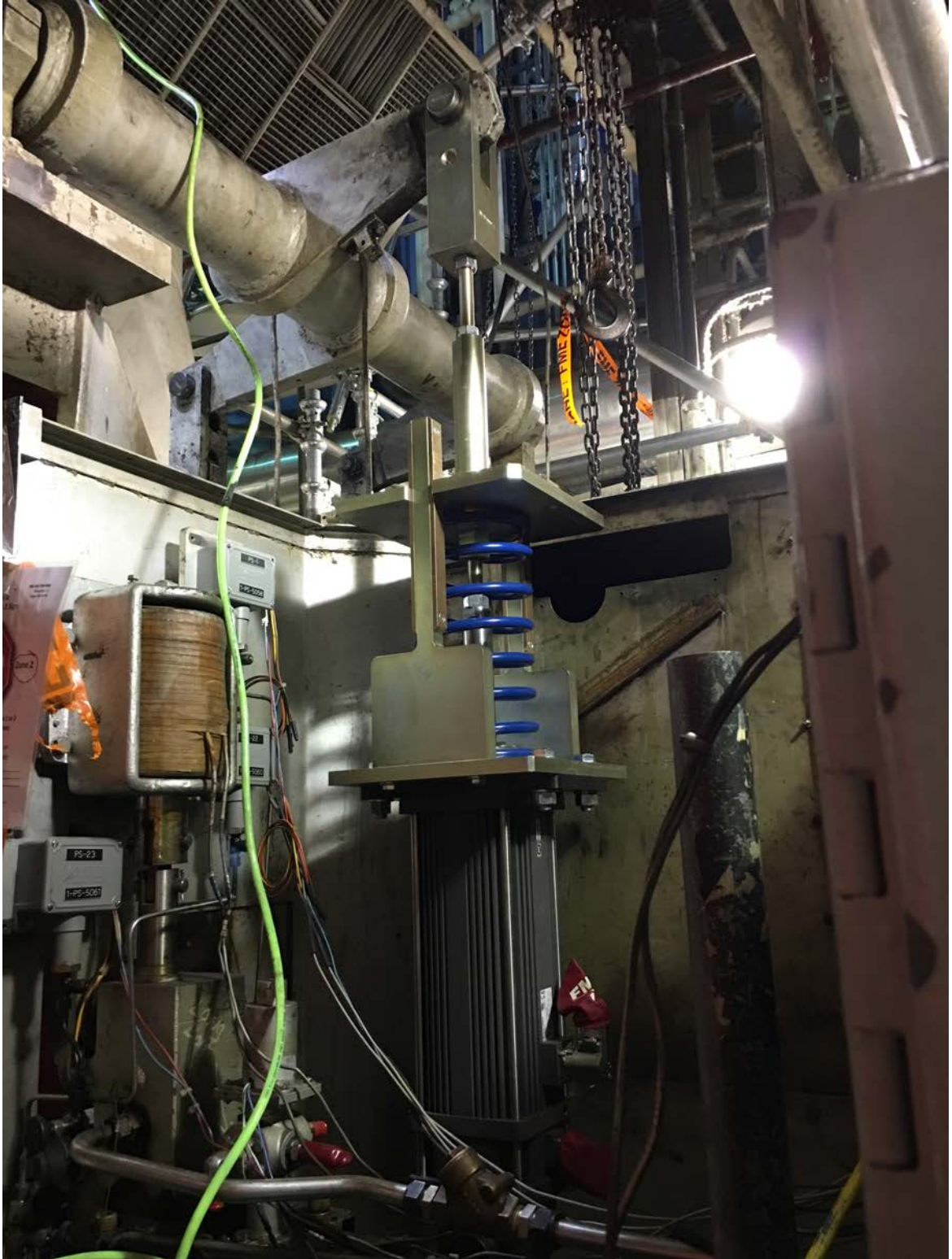
Figure 2. – Installed LP Electric Actuator Assembly
