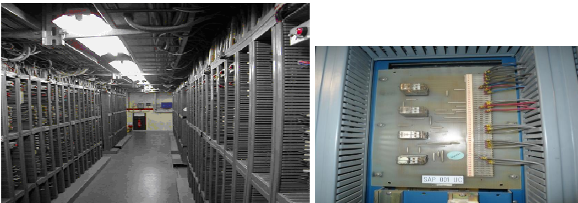
Figure 2: Relay racks and a relay module
